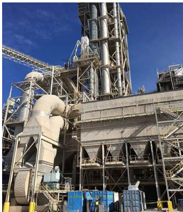
Sustainable Energy Solutions' Cryogenic Carbon Capture Demonstration. Demonstration plant at Argos Roberta cement plant (photo by Sustainable Energy Solutions).
